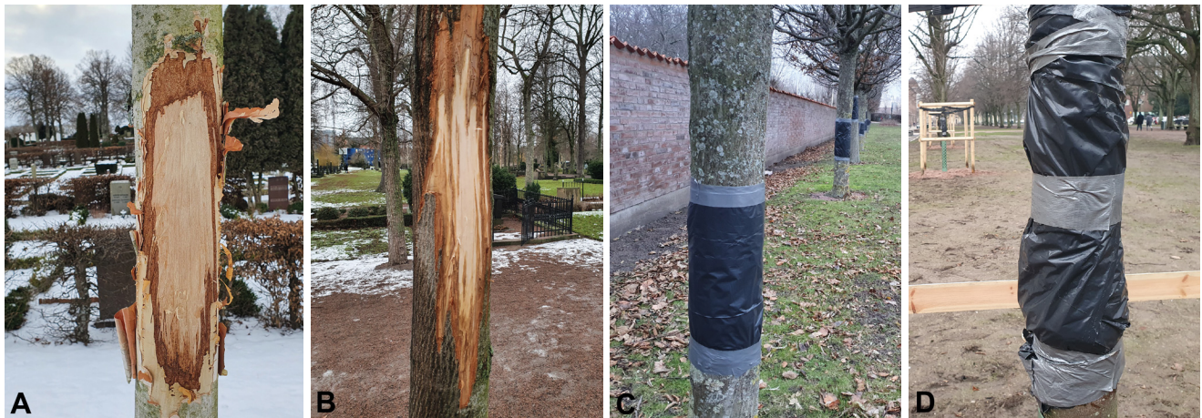
Figure 1. The photos (A) and (B) show trees located in the cemeteries with no plastic wrap. Here you can also see how the injuries typically looked. The photos (C) and (D) show trees located in the municipality with plastic wrap.
