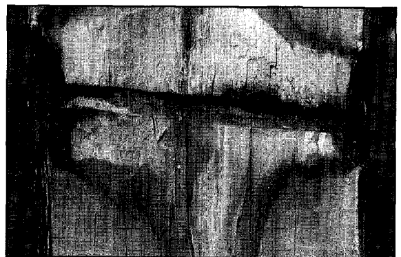
Figure 2. Some years after installation of a crown anchor: The bolt with a diameter of 18 mm (0.7 in.) led to discoloration and white rot above and below the drill hole.
