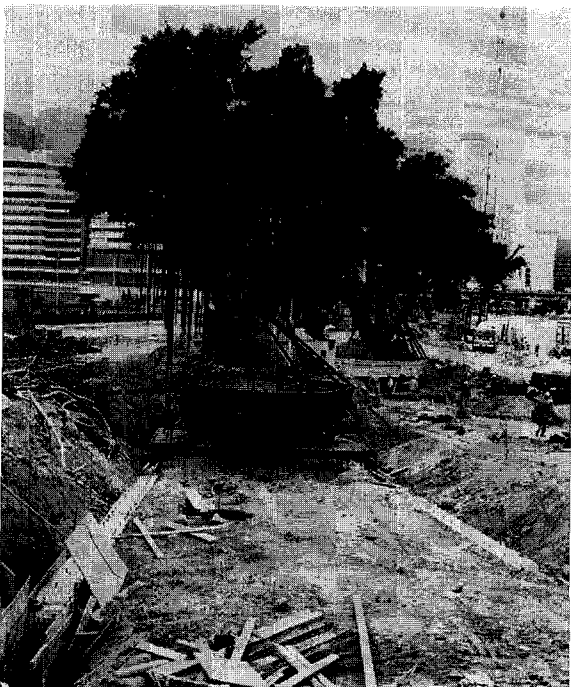
Figure 6. Tree A on the left and tree B on the right behind it immediately before the transfer. Note the construction of reinforced concrete rail bedding on which the tree would slide on rails towards the destination.
