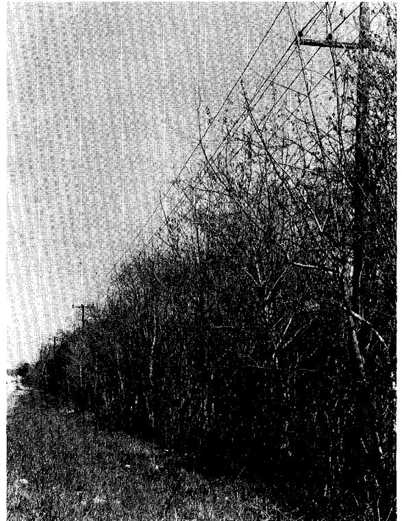
Fig. 2. A continuous maintenance problem exists where undesirable species have become established under distribution lines.
