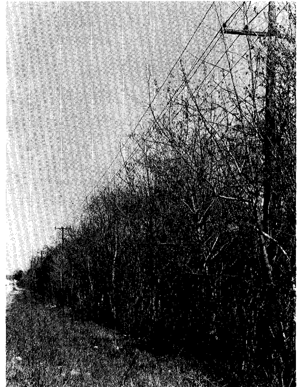
Fig. 2. A continuous maintenance problem exists where undesirable species have become established under distribution lines.
